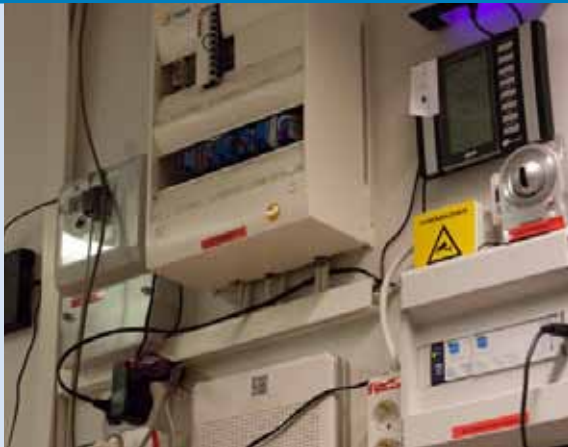
Monitoring equipment in smart housing
